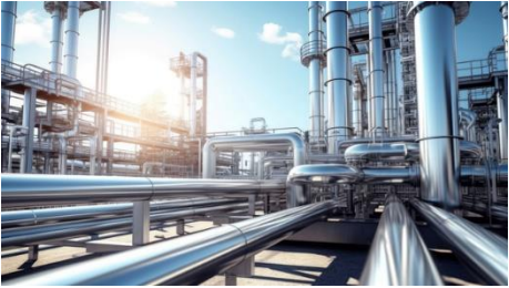
Gas supply line pipe
